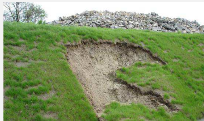
Example of shallow landslide
